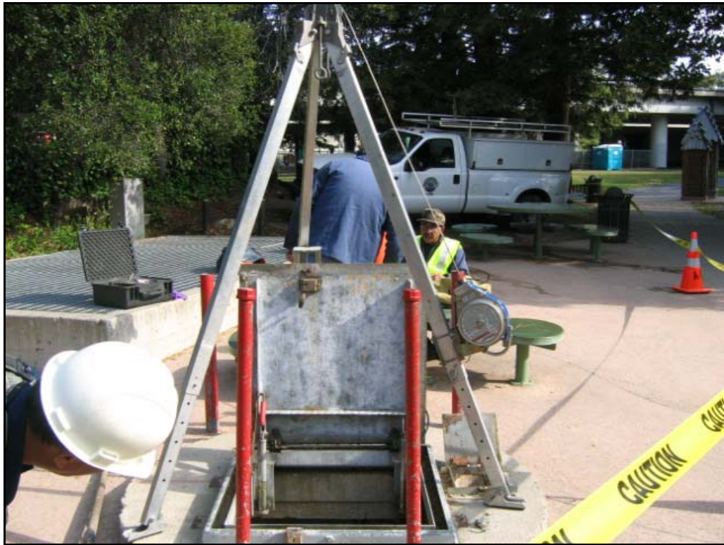
Figure 43: Getting the Pump ready for Potemkin Creek's summer flow. Photo by Jon Bauer.
